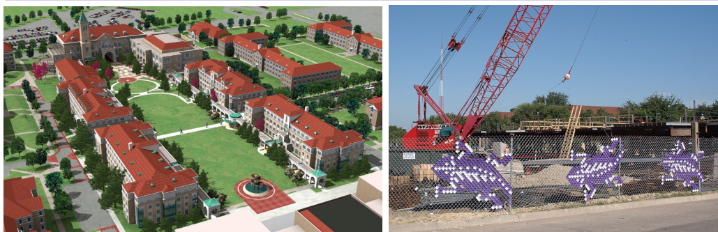
Dirt flies as the TCU construction continues throughout the 2006 school year. (Top and bottom right) Sight of construction in front of the Student Center. (Bottom left) Rendering of residents halls looking toward University Union.
