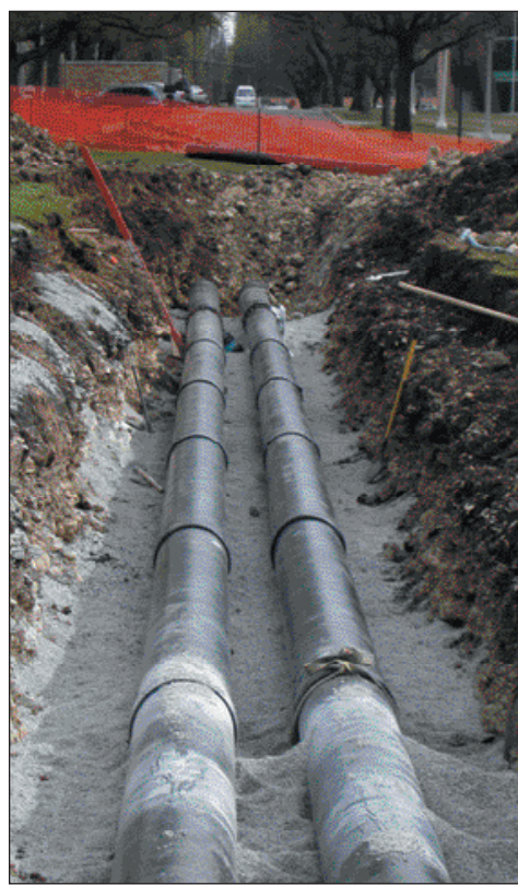
STEFANIE SHEFFIELD / Photographer Construction has started on pipes near Frog Fountain. The pipes are being moved to make room for a new residence hall.
